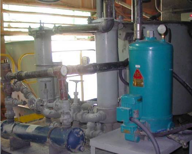
A CJC™ Fine Filter installed on Crusher 4 at Codelco Mine site in Chile
